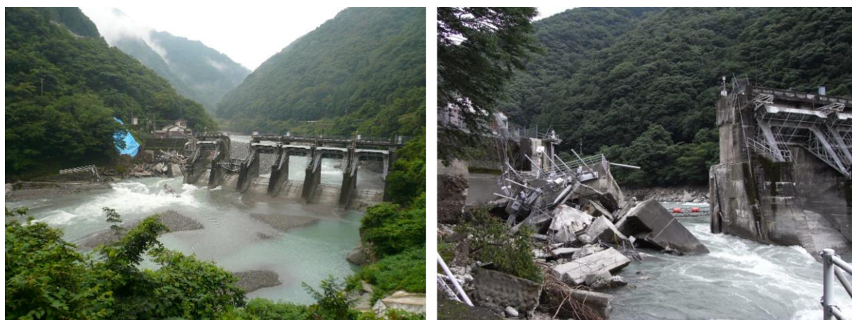
Figure 3-1 Flood Damage Cases at Kyushu EPCO's Kawabegawa No.1 Power Plant (Left: Damage to Intake, Right: Enlarged View of the Right Bank Slope)
