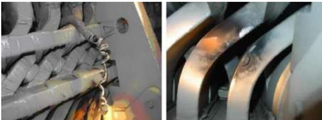
Figure 3-1 Stator bars with damaged insulation at ends
